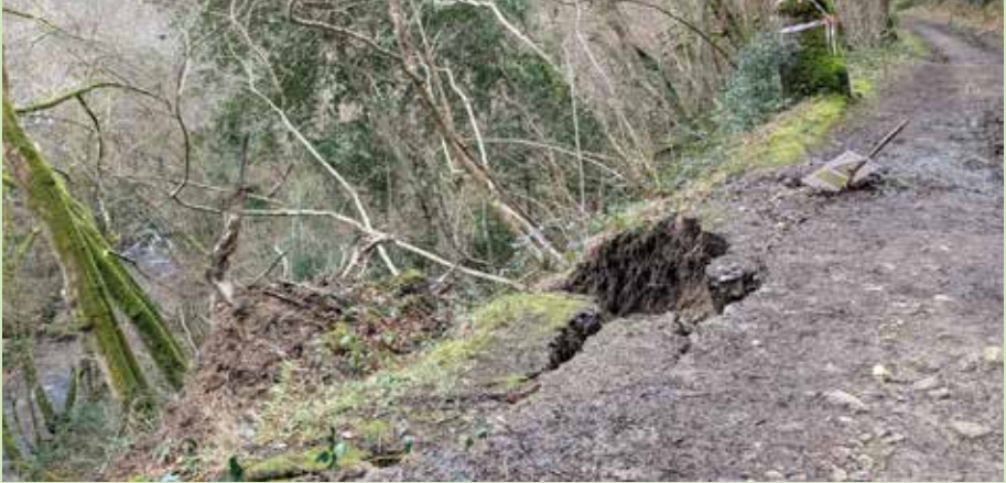
The fallen tree and the collapsed path
